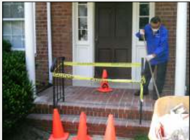
Nelson is seen repairing some of the mortar on the front stoop of 4317 S. 36th Street (Court 10).
