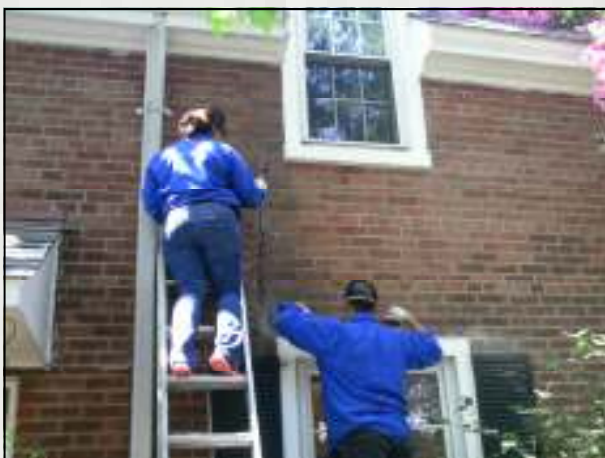
Nelson & Maria work together to repair mortar on the rear wall of 4343 S. 36th Street (Court 10).
