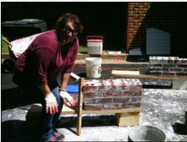
Maria completes her first project, which was learning to build solid walls and lay units in a line.
