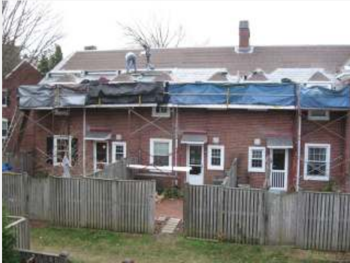
Workers for the roofing contractor replace a slate roof on S. Stafford Street as part of our roof replacement program.
