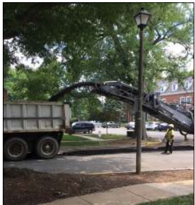
Crews from Arlington County work to mill this section of S. Stafford Street near Court 3. Once milling was completed, the asphalt paving crews moved in.
