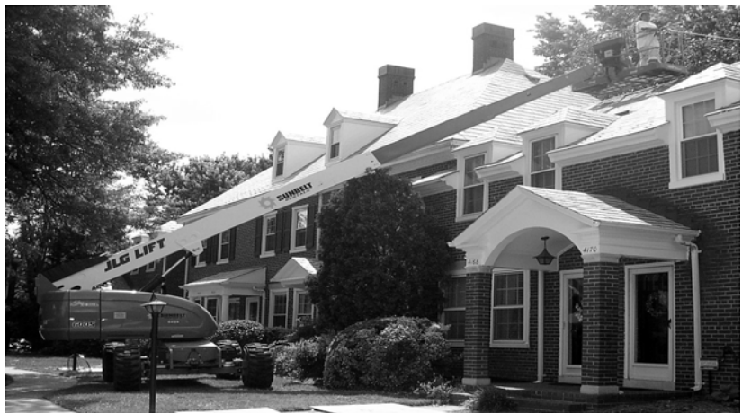
Pictured in Court 6 is an articulated manlift (manufactured by JLG Lift) being used by Middledorf Painting Company, our contractor. The lift is being used to ease the painting of upper elements of our buildings, and to minimize the need for placing ladders over our shingled roofs. This is the first time such equipment has been used for painting in the Glen.
