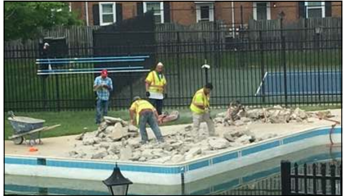
A portion of the concrete pool deck was sinking and needed to be replaced. A crew worked in April to dig up the slab.
