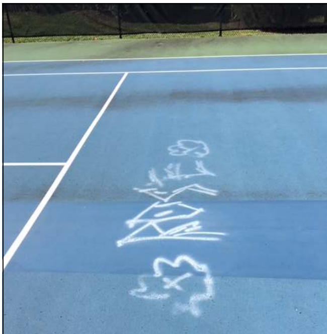
Examples of some of the markings made onto Glen property. Some of the markings have washed away in the rain, but others remain.
