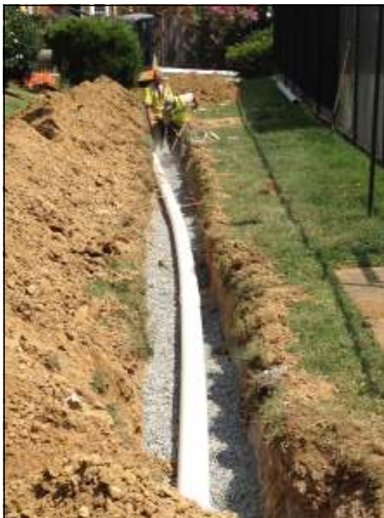
In early August, drainage work near the tot lot began. Here crews install a new pipe parallel to the tennis court.
