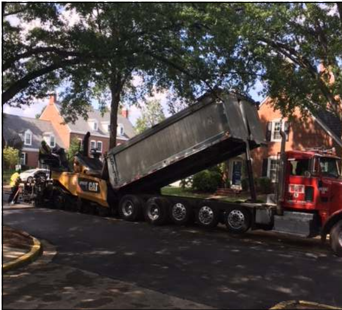
Hot asphalt is laid onto the street just in front of Court 14.
