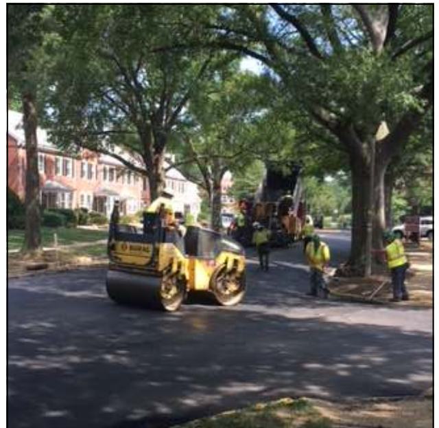
Then the road roller compacts the hot asphalt outside of Court 15 and creates a smooth surface.
