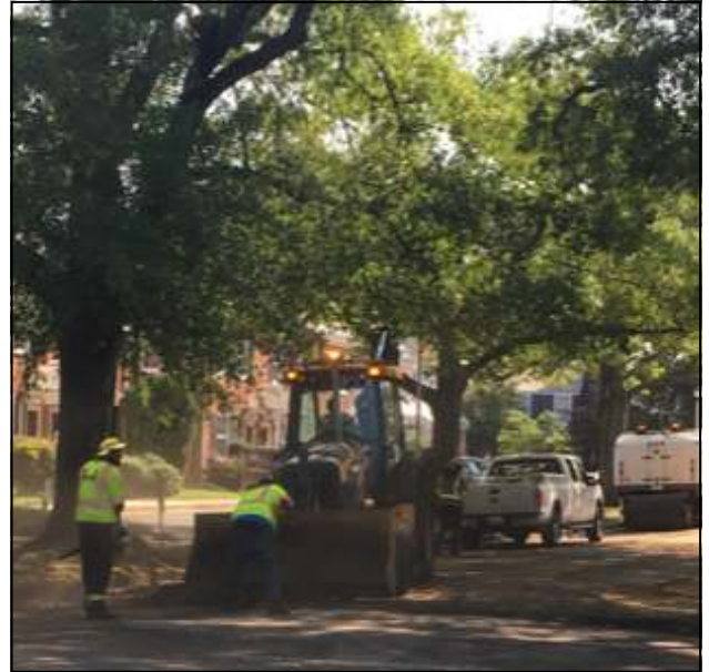
Crews arrive on August 29 and begin to get the street ready for new asphalt.
