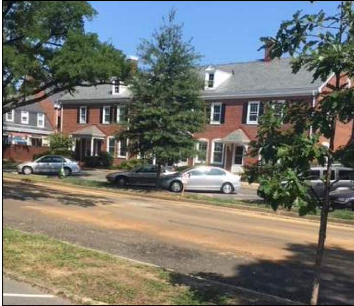
S. 35th Street after it was milled...just waiting for the paving crews to arrive.
