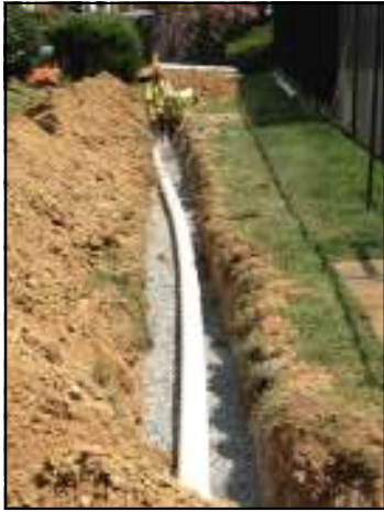
Sewer lines are part of our aging infrastructure.
