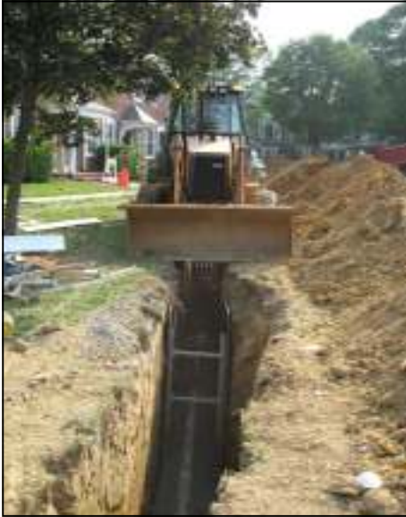
Construction workers dig a trench to reach one of the Glen's sewer lines. (file photo)
