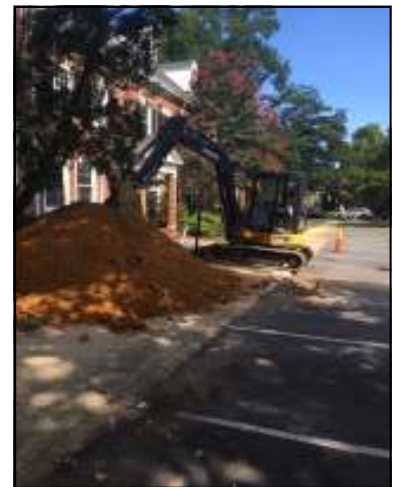
A large holly tree was removed as its roots caused the problem.
