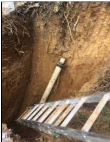
Dwyer Plumbing had to dig down deep in front of 3556 S. Stafford
