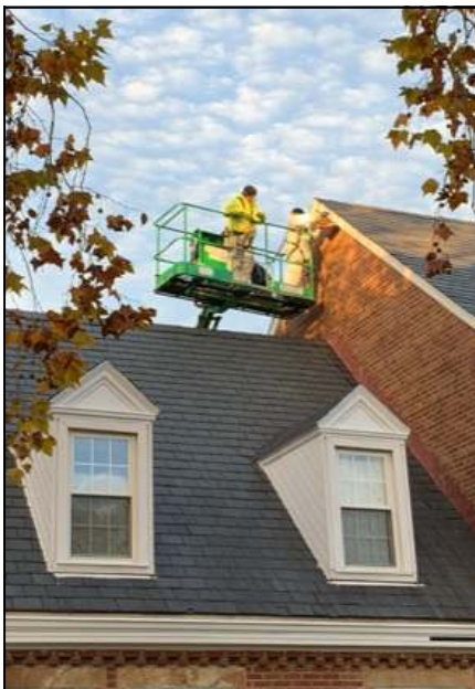
A crew from Williams Professional Painting works in Court 12 to paint the highest point of a building.
