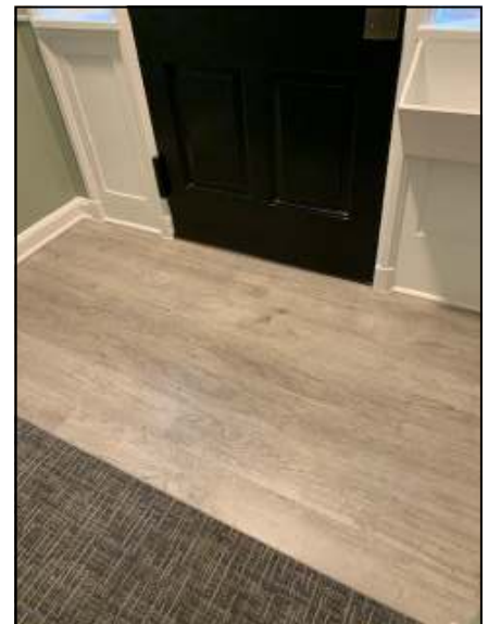
Just inside each B Building front door is a brand new luxury vinyl tile floor. Such an improvement!
