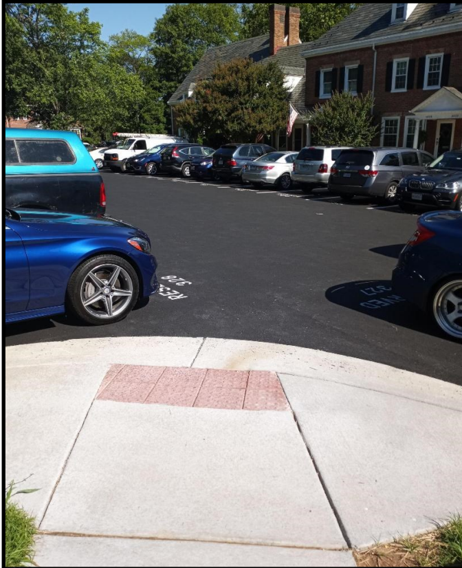
Court 10's parking lot was milled and repaved with new asphalt. The parking spaces have now been striped and numbered. And the lot remains handicapped accessible.
