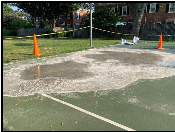
This depressed area of the Glen's basketball court is readied for repairs. (photo by Mary Bley)
