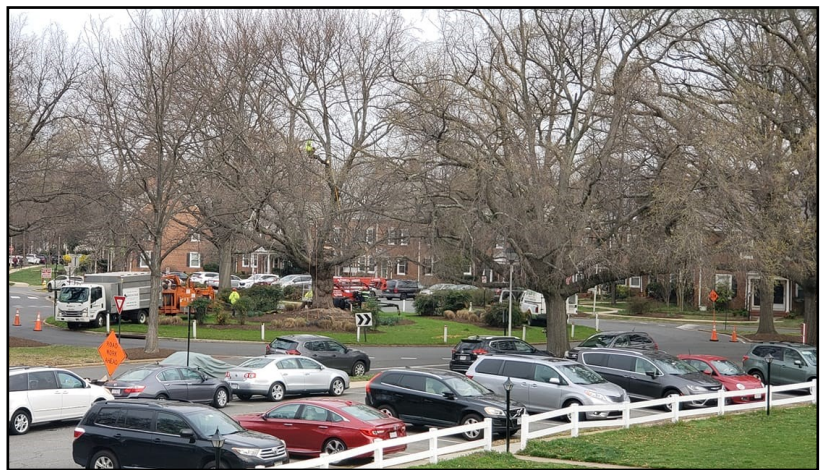
Crews work on the tree in the S. Stafford Street circle. Photo shows the scene from Court 4.
