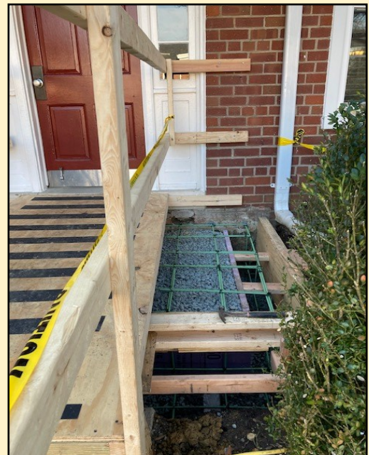
Crew members have installed a temporary ramp to access the B Building.
