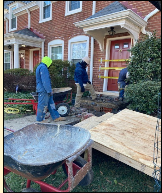
Crew members examine the foundation at 3555 S. Stafford Street after demolishing the existing stoop.
