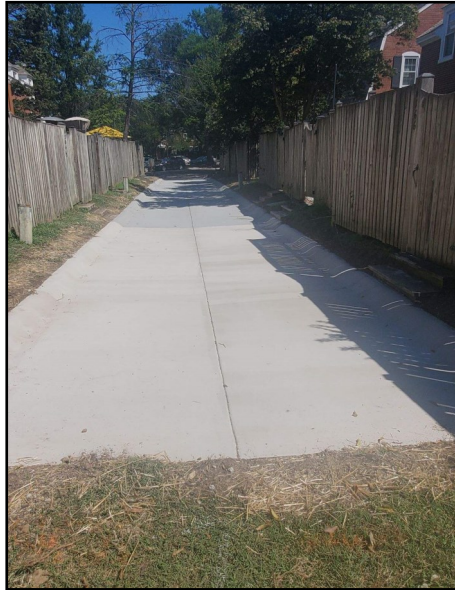
Finished product! The Court 6/7 alley with its new concrete curbs and pads.
