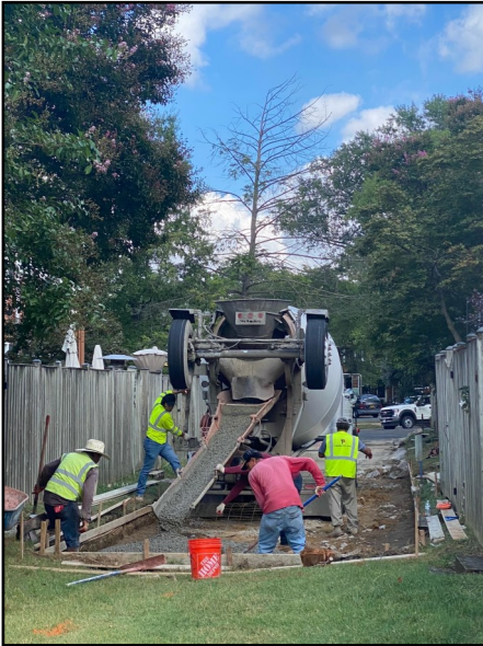
Crews from Dominion Paving begin to pour concrete in the Court 6/7 alley.
