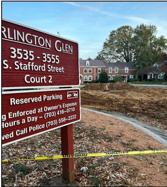
The yellow caution tape was out in Court 2 as the lot was closed for several days for full replacement.
