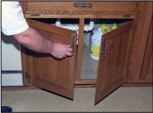
This allows heat to reach the pipes.
