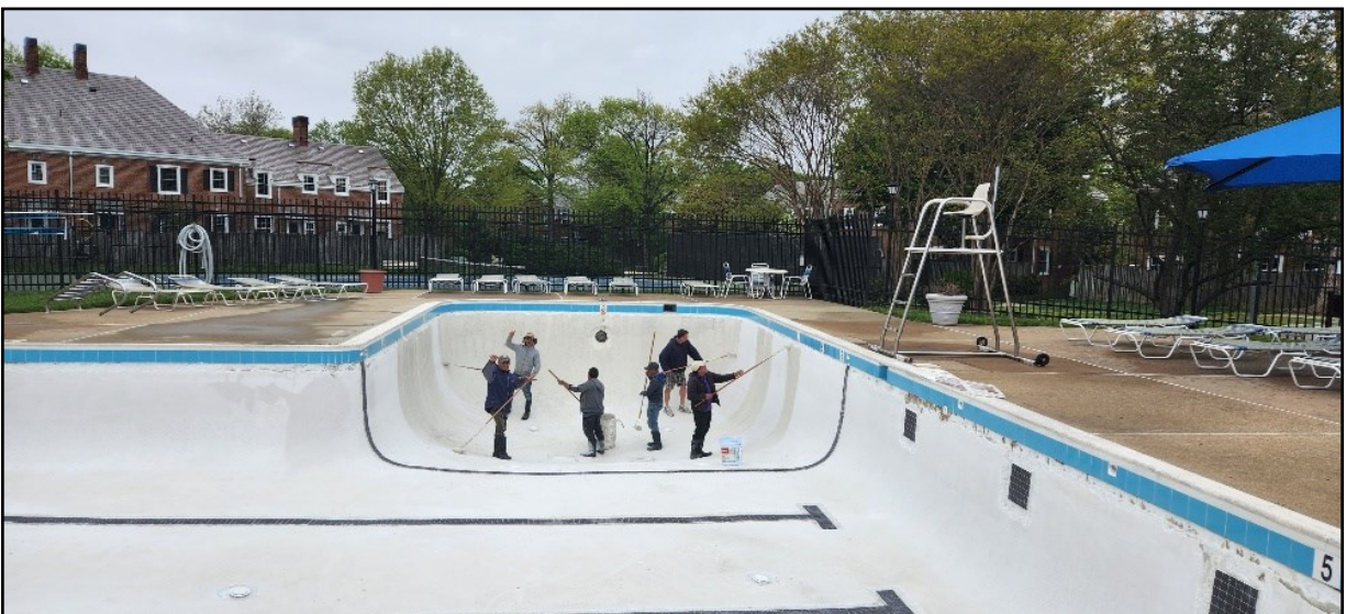
Our pool contractor, Atlantic Pool Services, Inc., has completed any repairs and whitewashing to both the main pool and the baby pool so the surfaces will be smoother on your feet.
