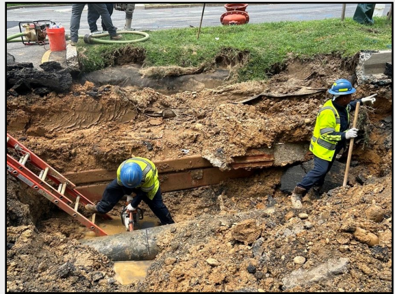
County crews work to repair a water main break in the Four Mile Run area on June 7, 2024.
